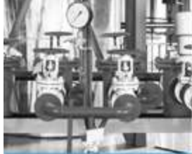
UPSTREAM / PROCESS WATER TREATMENT
